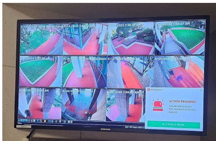
Courthouse Camera Monitors
