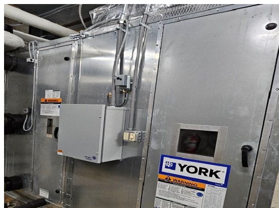
Building Mechanical Repairs and Improvements - Air Handler
